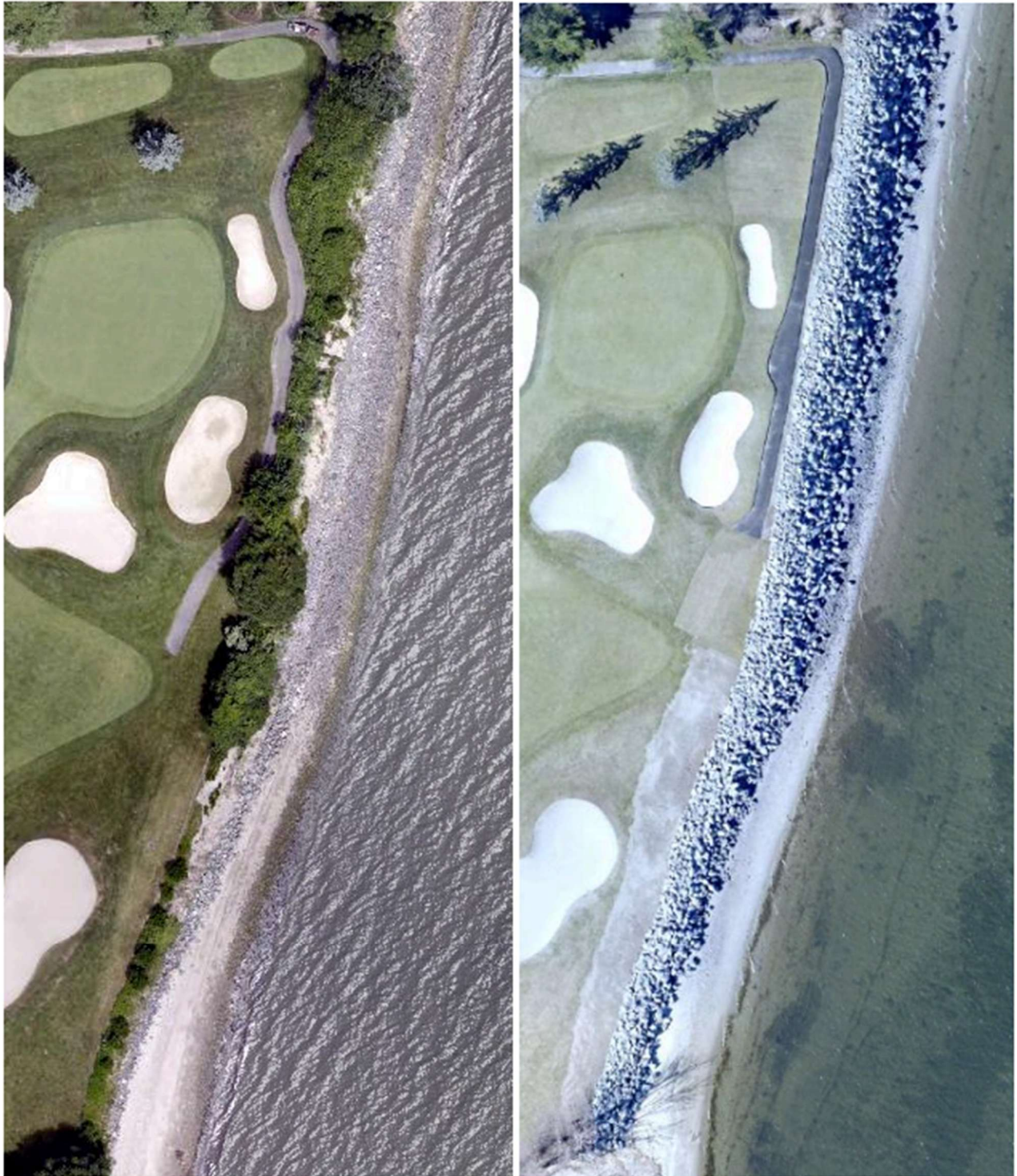
Figure 2: Photo Comparing the Coastal Features Before and After the Riprap
